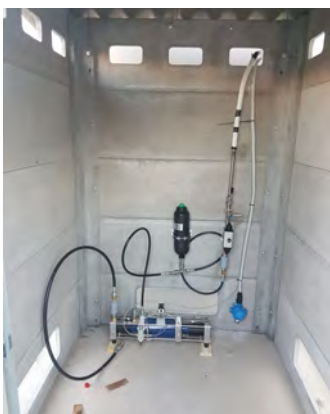
1. Supply Room Refrigerant transfer pump (RTP)
