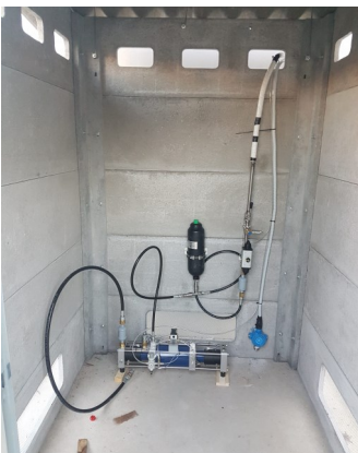
1. Supply Room Refrigerant transfer pump (RTP)
