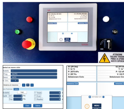
Touch screen machine Controller
